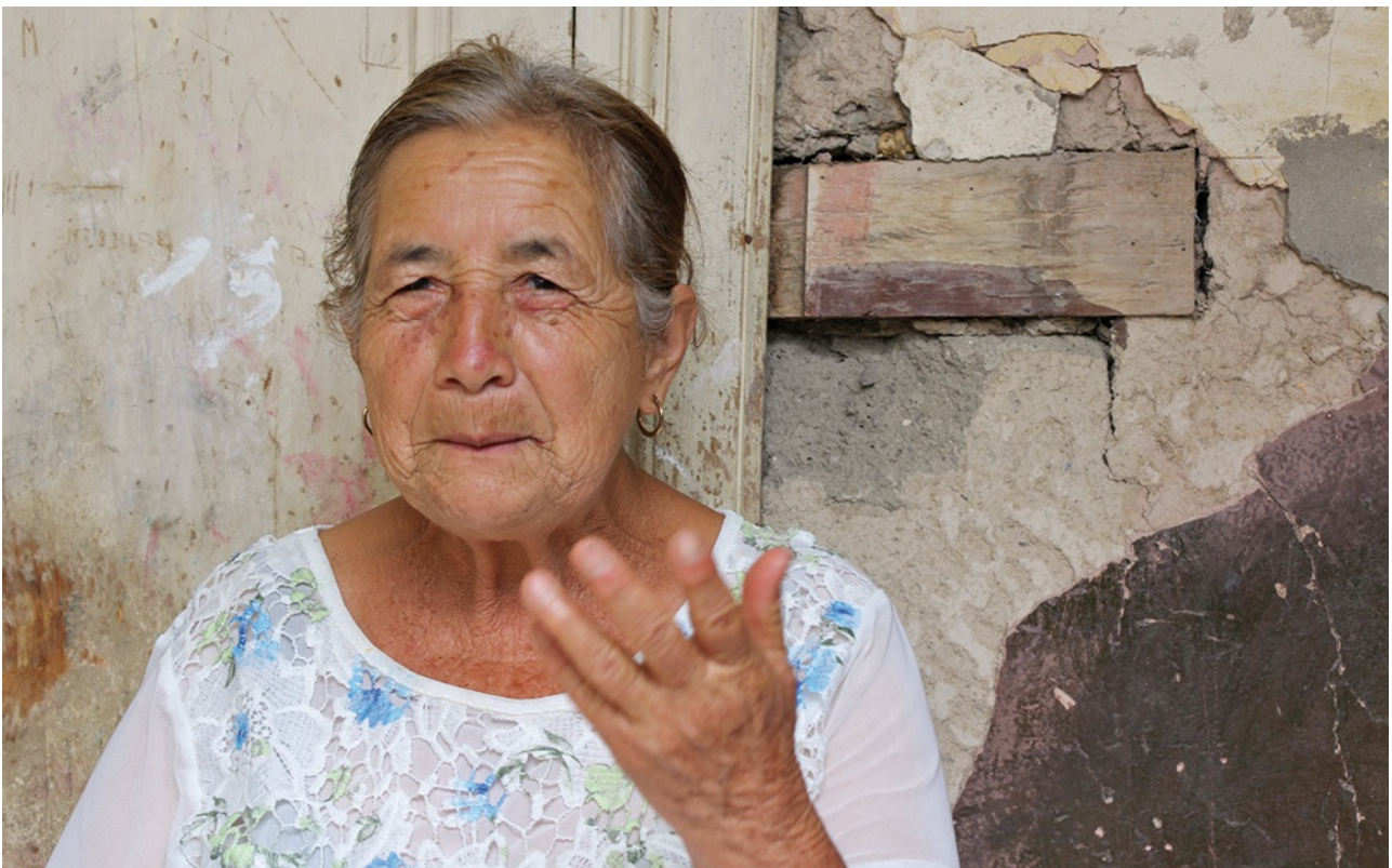
Carmen Cecilia Acuña lives in a very old and deteriorated house in Soata, Colombia. Her house is made of mud and the roof is made of cane, a haven for triatomine bugs. When the municipality inspected her house, it found more than 60 triatomine bugs. They fumigated the house and tested the entire family. Carmen was the only one to be tested positive for Chagas disease.
